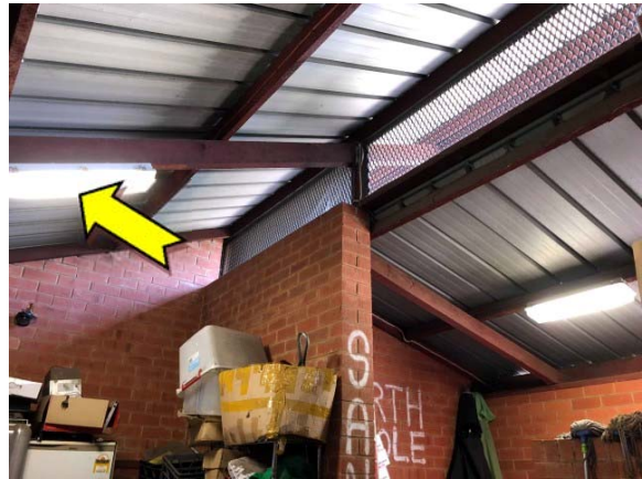
Photo 4. Interior, store room, double tubed fluorescent light fittings – suspected PCB-containing capacitors.
