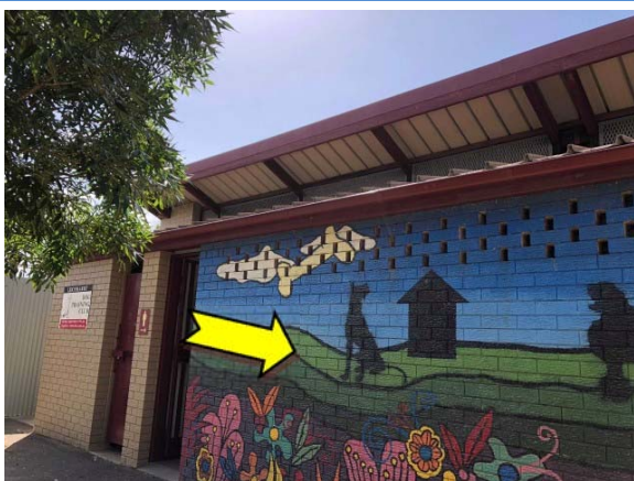
Photo 5. Exterior, throughout, graffiti wall – suspected lead-containing various upper coloured paint systems.
