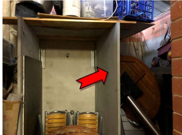
Photo 2. Interior, north elevation, store room, shower partitions – asbestos-containing fibre cement.
