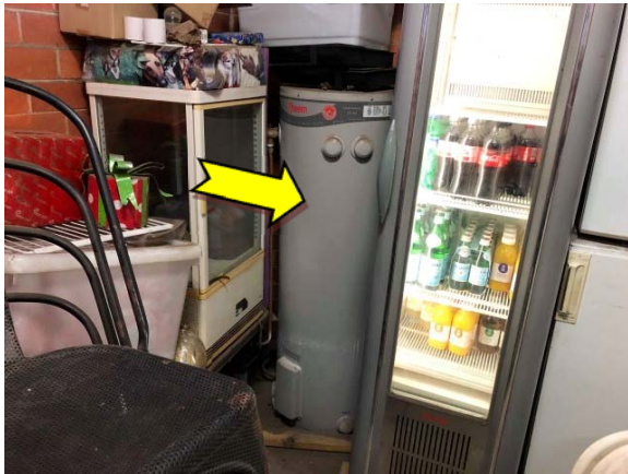
Photo 3. Interior, south-east elevation, store room, hot water heater – suspected SMF internal insulation material.
